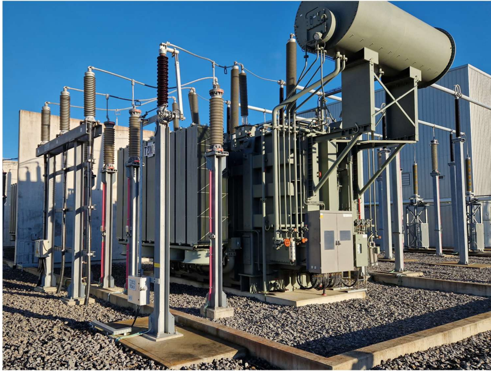
Figure 3: Typical Transformer and Outdoor Equipment.
